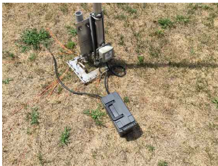
Remote tuner located at the base of the antenna for testing purposes. Upgrades in the future.
